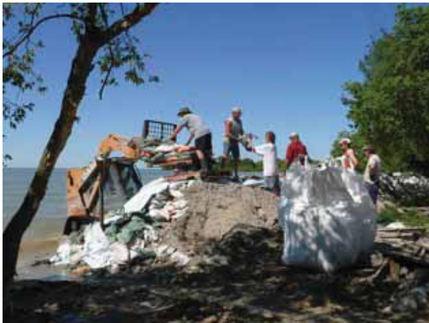
Raising a dike, and securing the poly. At night, and when winds are high, skidsteer access places are blocked by 'super sandbags'. Each weighs 1500 - 2000 lbs.
